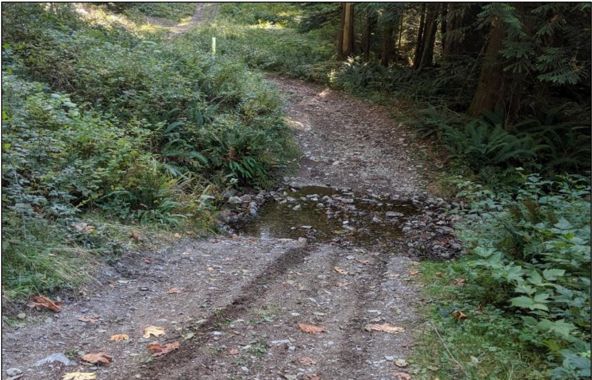
Photo 1: Ford crossing the natural gas pipeline road, without erosion sediment and control structures and no means to prevent recreational use.
